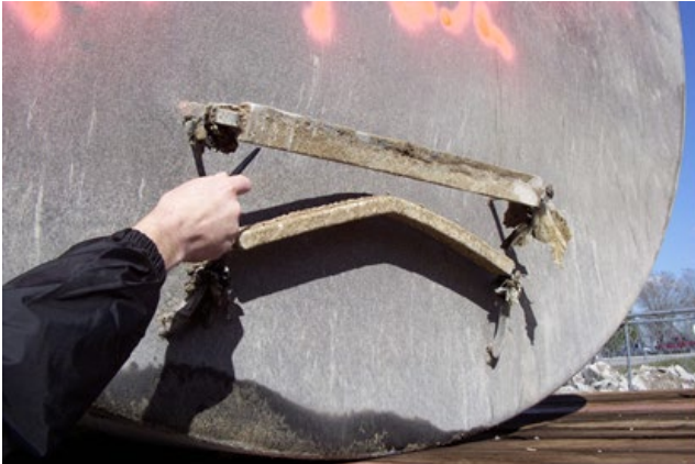
Steel Tank with anode
