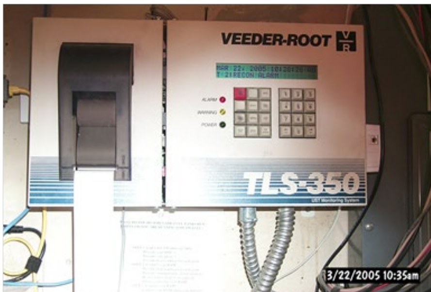
Example of an ATG monitor
