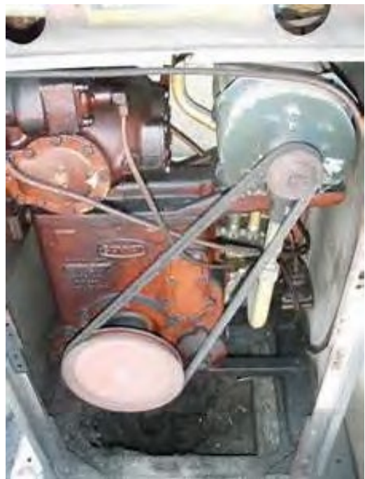
pump under dispenser - suction
